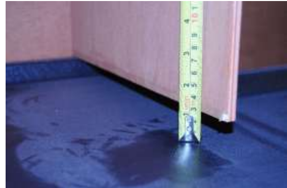
Figure 28: The partition wall above this removable floor poses an entrapment risk
